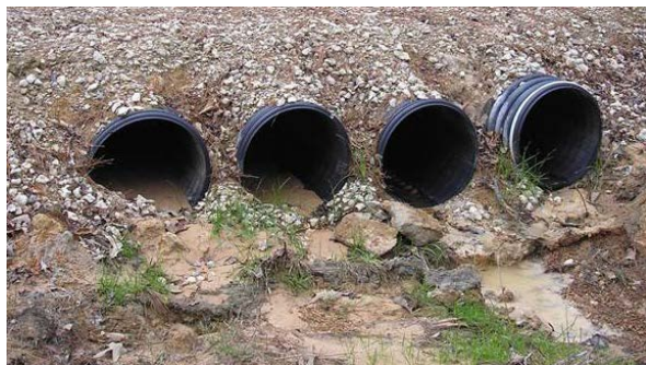
Figure 2-12: Culvert erosion—early-stage gully/rill erosion between the culverts
