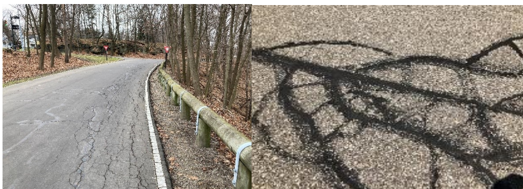
Figure 2-8: Pavement and shoulder alligator cracking
