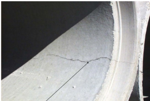
Figure 2-32: Longitudinal crack within a concrete barrel
