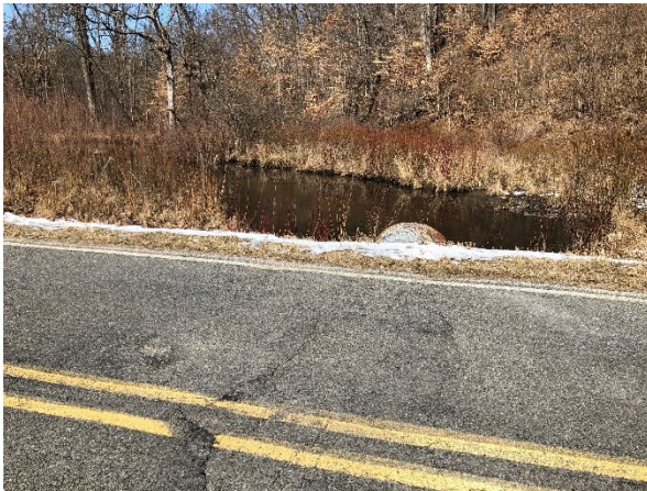
Figure 2-6: Transverse cracking of pavement above culvert
