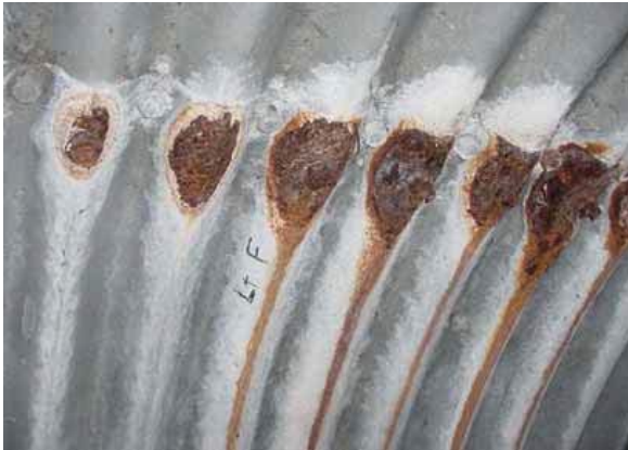
Figure 2-35: Corrosion of a metal culvert
