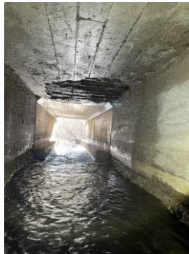
Significant soffit spall with exposed reinforcement
