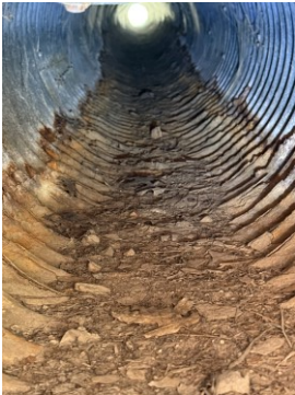
Uniform corrosion loss along invert. Wall penetration possible with pick
