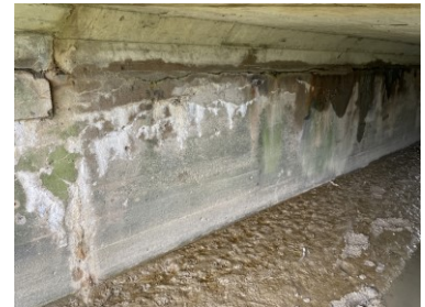
Hairline to wide cracking along culvert soffit
