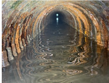
Localized deep pitting
