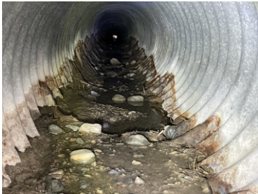
100 percent section loss along invert
