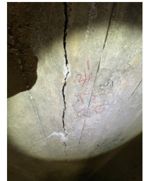
Wide longitudinal cracking along soffit
