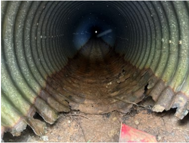
Moderate corrosion with minor section loss throughout barrel
