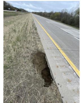
Sinkhole undermining roadway
