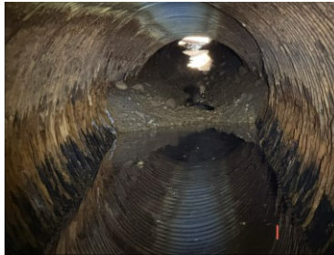
100 percent section loss along invert with backfill migration
