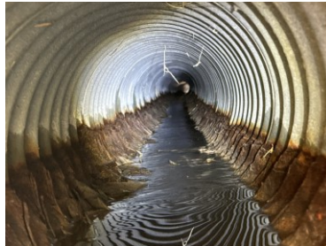
Moderate corrosion along invert (perforations visible and easily made)
