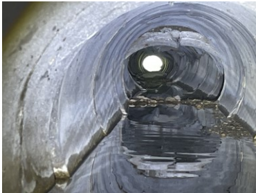
Barrel failure beneath embankment
