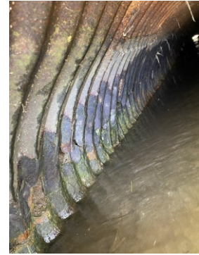
Culvert sidewall buckling and section loss
