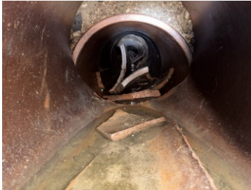
RFA Priority level 1: Barrel failure under roadway
