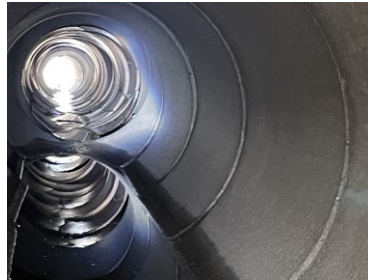
Structural cracking and barrel misalignment beneath roadway depression
