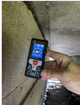
Three-sided culvert wall rotation
