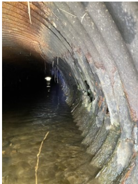
Culvert sidewall buckling and section loss
