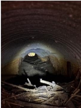
100 percent section loss along invert with backfill migration
