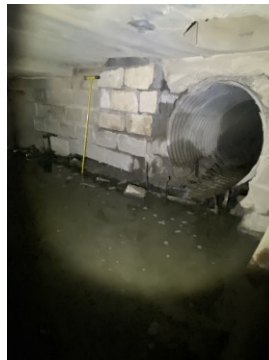
Culvert wall block displacement
