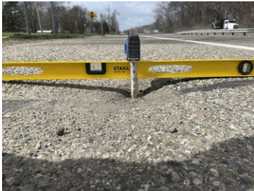
Sinkhole in asphalt shoulder
