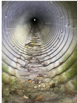
Visible section loss with perforations of CMP
