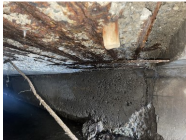
Moderate concrete section loss exposing steel reinforcement
