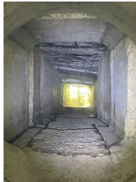
Soffit spalling exposing reinforcement
