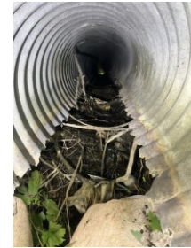
Invert section loss beneath roadway
