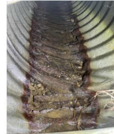
Localized section loss less than 1 inch in diameter
