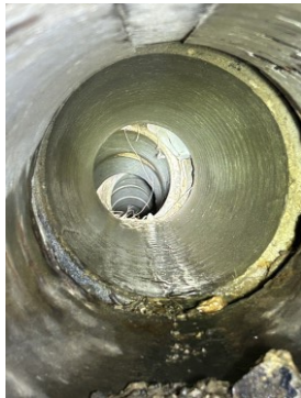
Joint failure with sediment infiltration through joints
