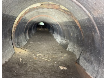
RFA Priority level 2: Joint separation with backfill infiltration
