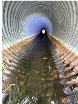
Isolated section loss beneath embankment
