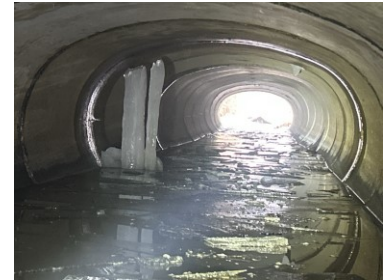
Active water infiltration through culvert joints within embankment
