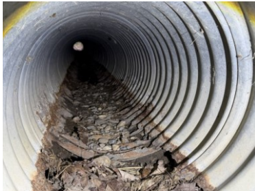
Visible perforations near end treatment
