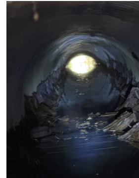
Invert section loss beneath roadway
