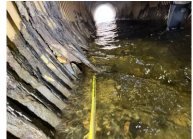
Isolated areas of full section loss
