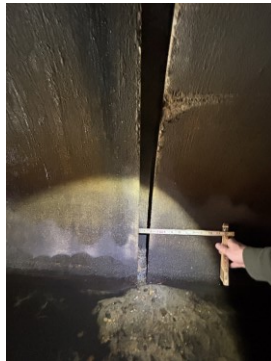
Wide joint separation with coarse grain infiltration
