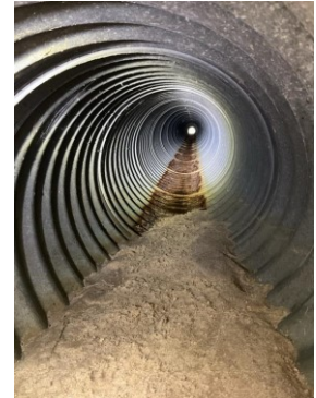
Corrosion along invert with holes less than inch in diameter
