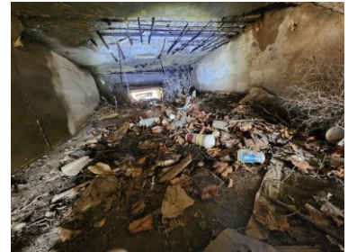
Significant section loss exposing reinforcement
