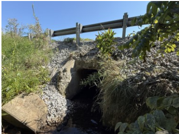
Failed wingwall with active embankment erosion
