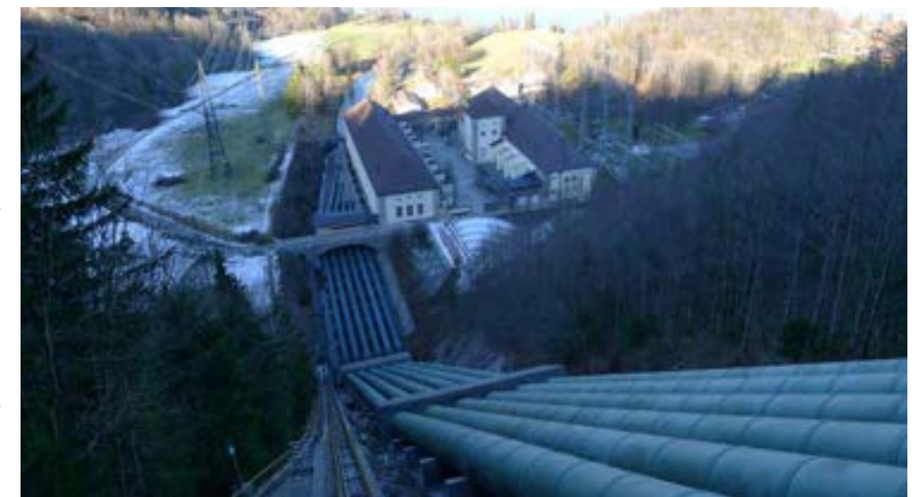
Penstocks at Walchensee power plant
