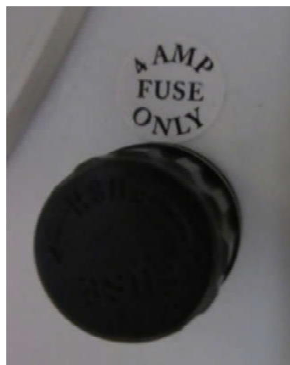
Vent fuse PHOTO F-1
