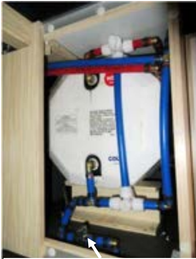
Drain valve PHOTO G-3
