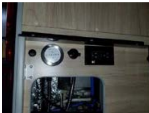
Utilities under bench-bed PHOTO E-34
