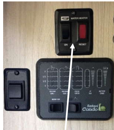
15 L Propane water heater switch PHOTO D-9
