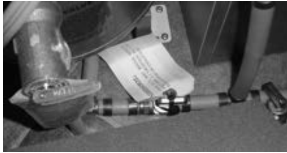
Hot water shut-off valve PHOTO G-2
