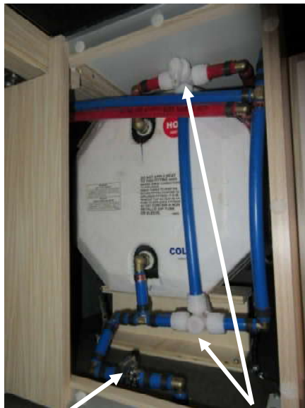
1 2 Drain valve and bypass valves PHOTO D-10
