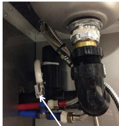
Water supply valve (XL FLEX) PHOTO G-7
