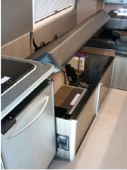
Motor under bench PHOTO E-47
