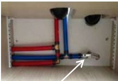
Cassette toilet valve under sink PHOTO D-30
