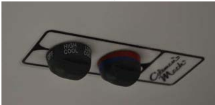
Circulation switch and thermostat PHOTO F-8
