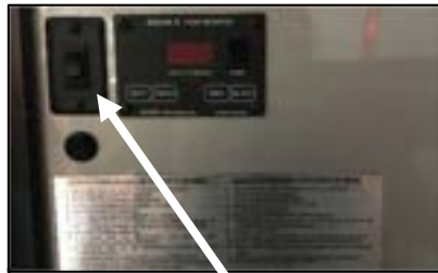
PHOTO K-21 Roof control switch
