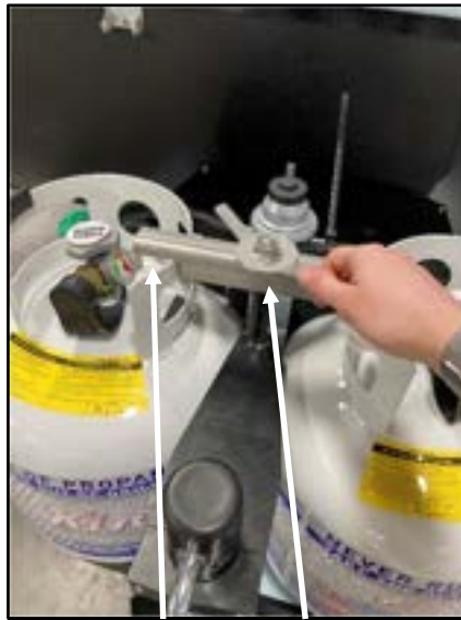
2 1 PHOTO G-4 Double propane tank mount
