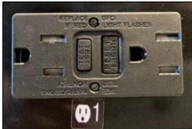
PHOTO H-1 Electrical outlet with GFCI
