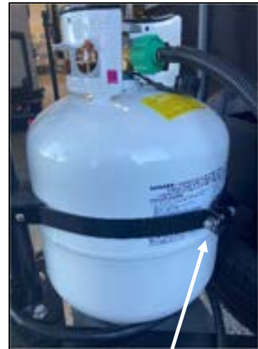
PHOTO G-3 Single propane tank retaining bolt
