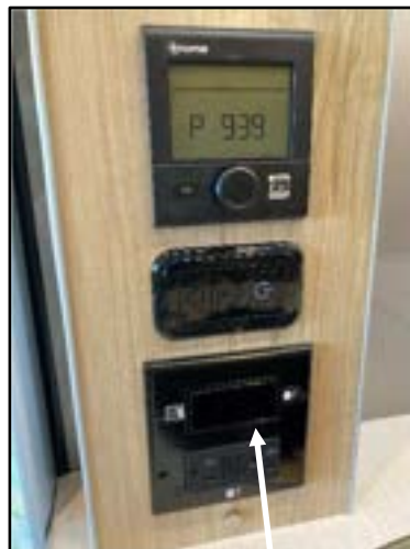
PHOTO H-4 Outlet #1/microwave selector switch
