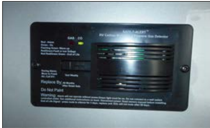
PHOTO B-2 Carbon monoxide and propane gas detector
