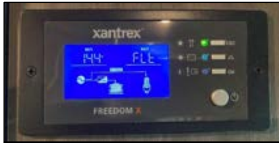
PHOTO H-3 Inverter control panel
