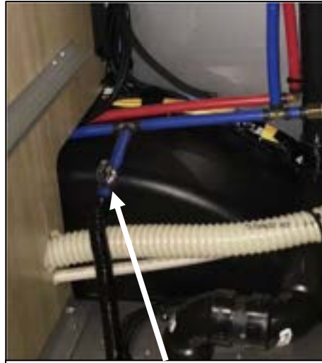
PHOTO K-3 R Series - Plumbing valve
