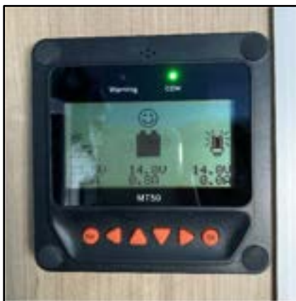
PHOTO J-2 Solar panel monitor
