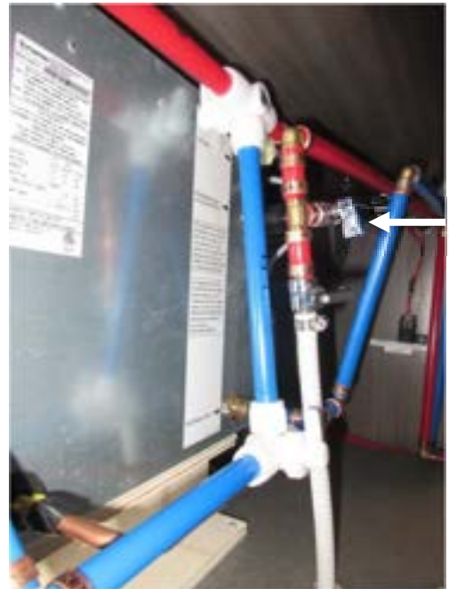
PHOTO D-10 Valve E
