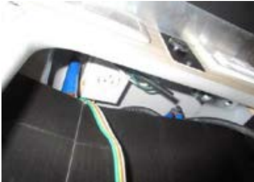
Water heater wall plug PHOTO D-4
