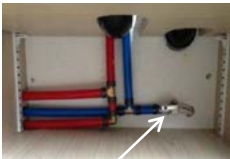
Cassette toilet valve under sink PHOTO D-30
