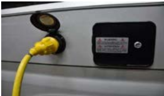
Power hook-up PHOTO C-1
