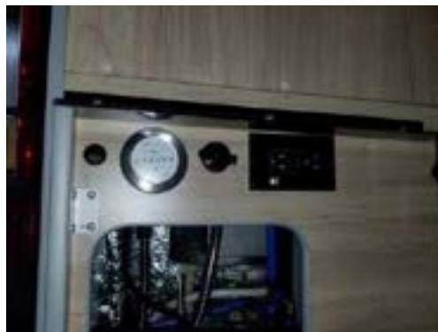
Utilities under bench-bed PHOTO E-34
