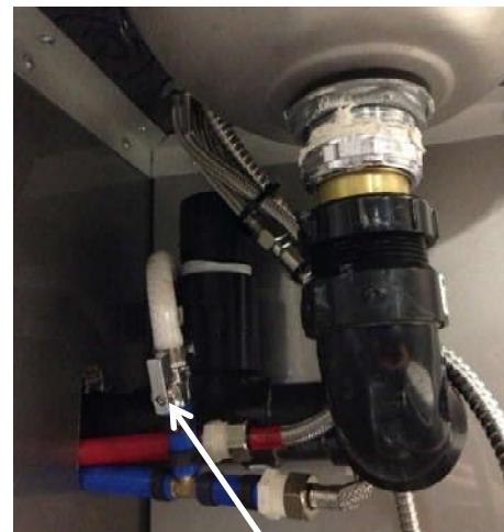
Water supply valve (XL FLEX) PHOTO G-7
