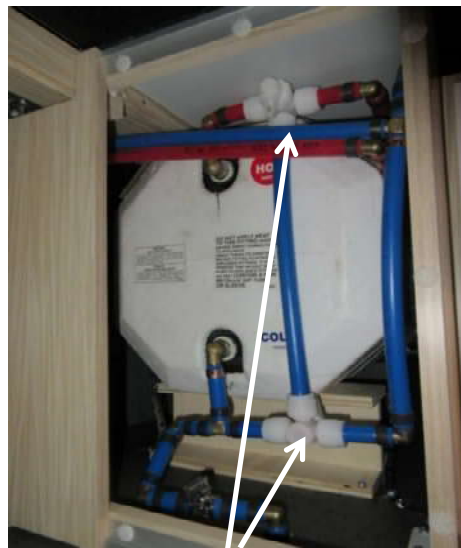
Winterizing valves (propane water heater) PHOTO G-5
