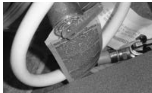
Safety valve PHOTO D-6
