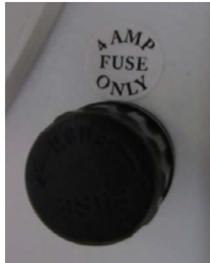
Vent fuse PHOTO F-1
