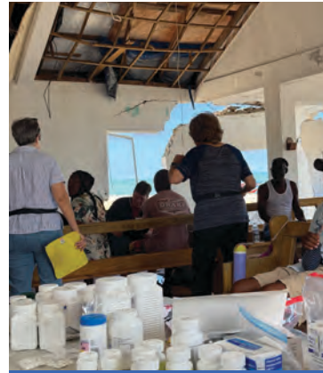
A makeshift clinic in a church damaged by Hurricane Melissa.
