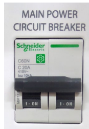
[Circuit breaker ON]
