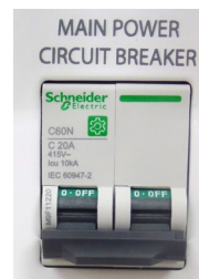
[Circuit breaker OFF]
