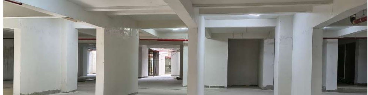
▲ Basement VDF flooring
