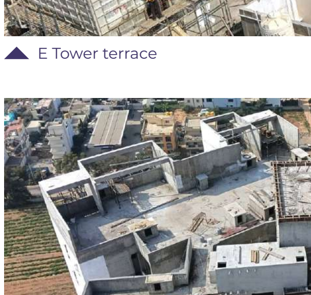
▲ Terrace domestic water storage tank
