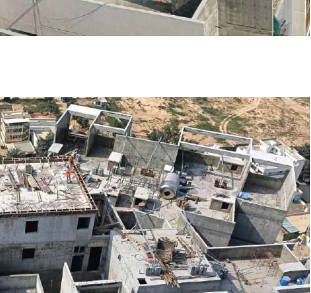
▲ Terrace recycled flush water storage tank
