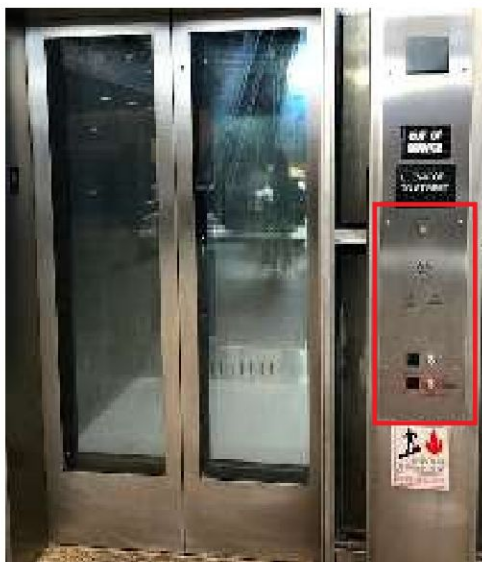
Installed Elevator with SIP Kit
