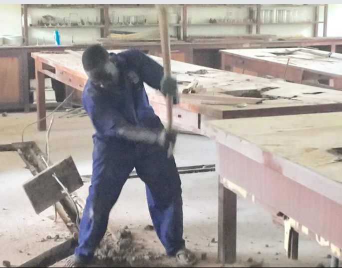
SHS Science Lab renovation – removing old gas lines buried in the floor.
