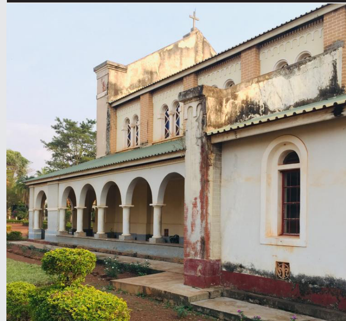
SHS worship space requires maintenance.
