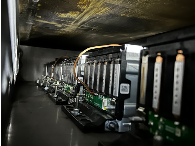
Sample: 2024408 - Picture #15 Battery housing with modules inside the rack
