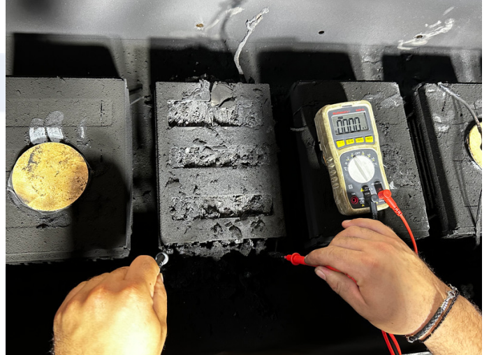
Sample: 2024407 - Picture #8 Ignited module, destroyed by the thermal runaway
