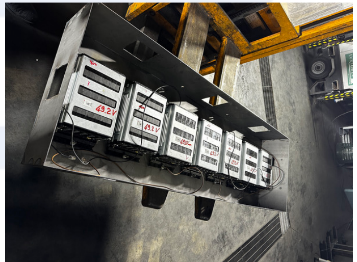
Sample: 2024408 - Picture #14 Modules positioned inside the battery housing
