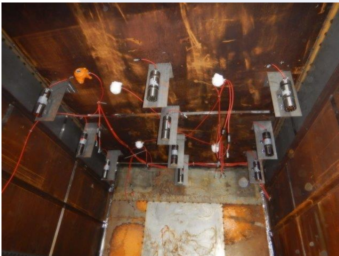
Sample: 2024408 - Picture #13 Extinguishing system
