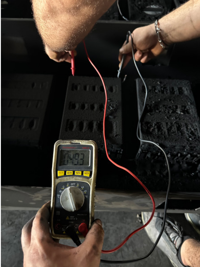
Sample: 2024408 - Picture #20 Surrounding modules still working after the test
