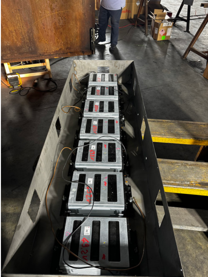
Sample: 2024407 - picture #1 Modules positioned inside the battery housing
