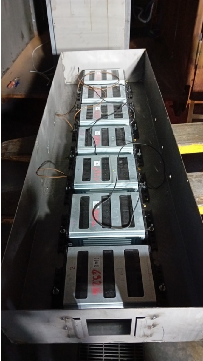
Sample: 2024408 - picture #11 Modules positioned inside the battery housing
