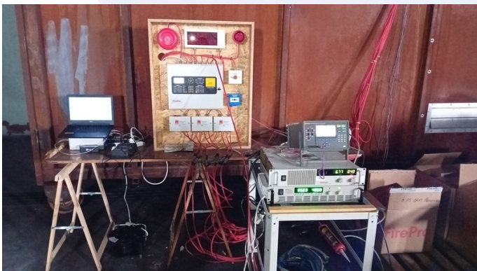
Sample: 2024408 - Picture #17 Control panel and instrumentation equipment
