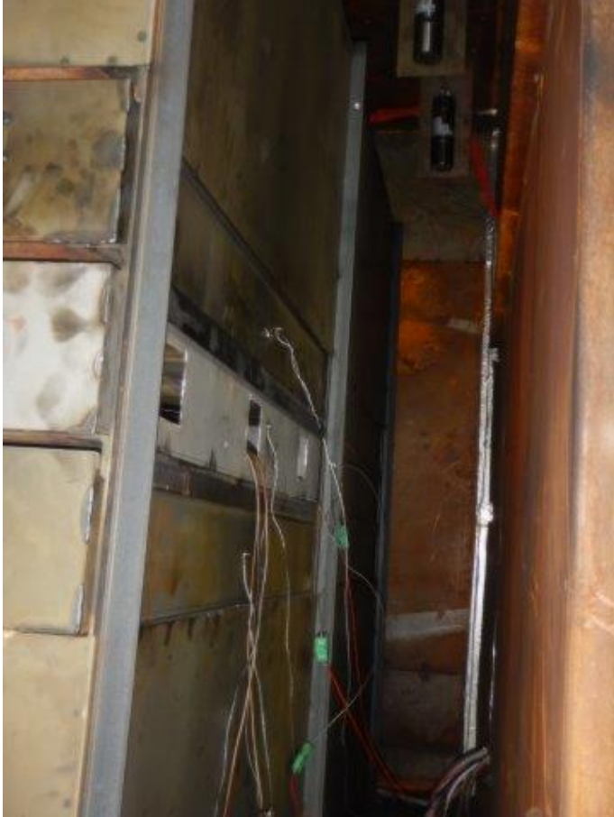
Sample: 2024408 - Picture #18 Thermal probes
