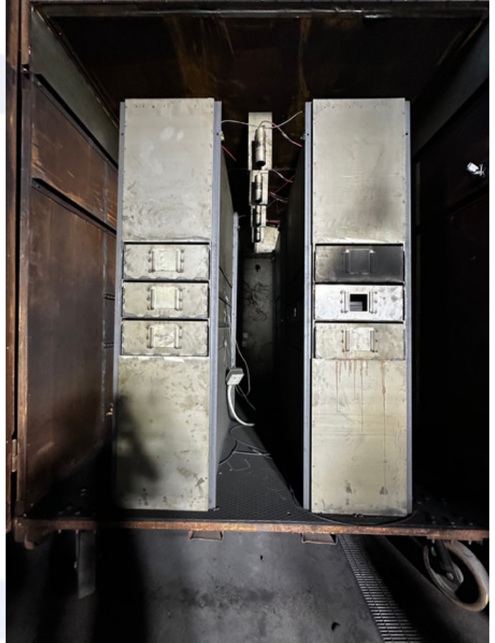
Sample: 2024408 - Picture #16 Racks ready for the test
