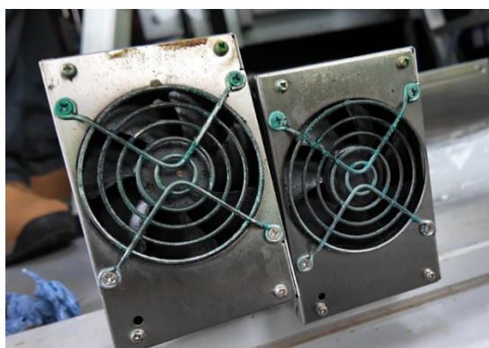
Fig 2 – Corrosion / Discolouration caused by prolonged (12 weeks) exposure to condensed aerosol without any post discharge actions.
