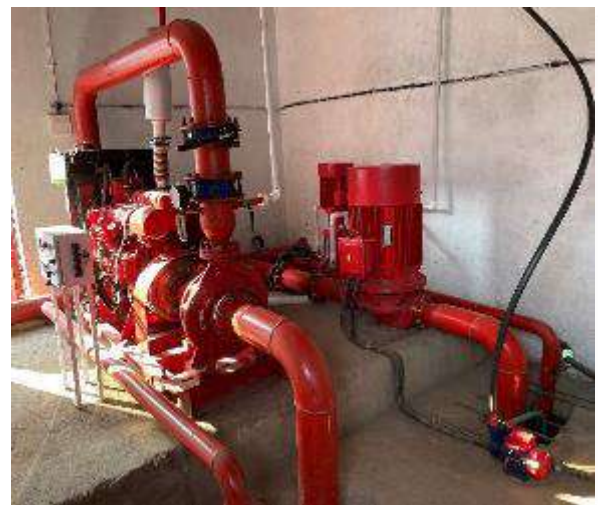
Operational fire pump room
