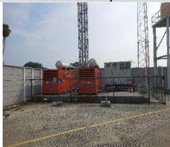
Diesel Generator Space
