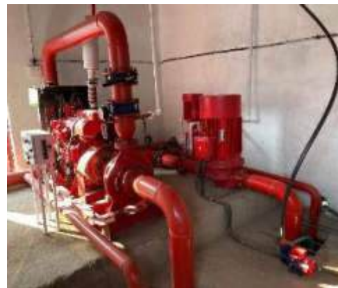
Operational fire pump room
