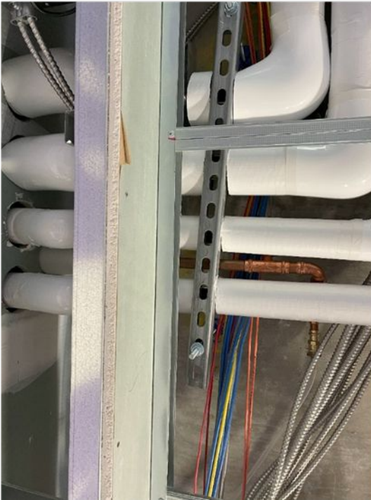
Continuous Insulation at Hangers
