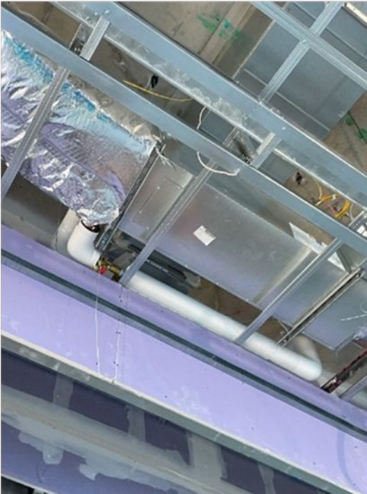
Inaccessible Access Panels
