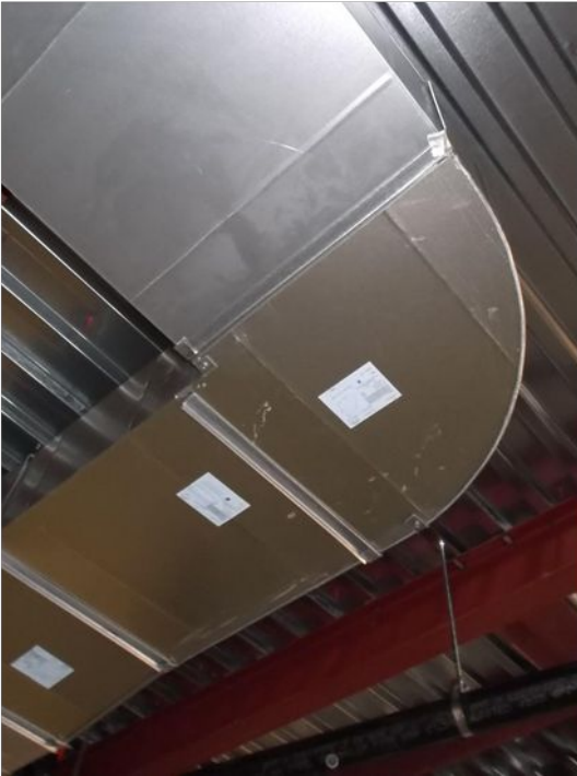
Improper Duct Transitions
