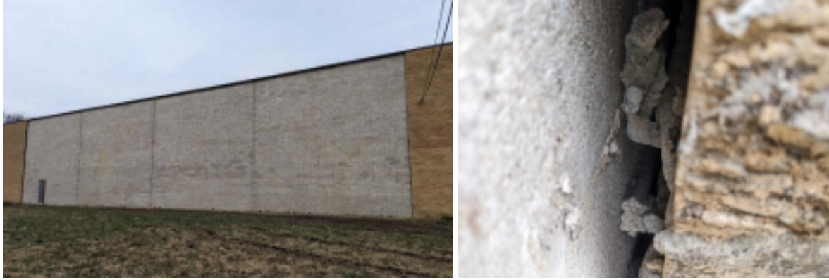
Collapsed veneer removed, exposing the CMU backup wall. Deteriorated and broken corrugated steel masonry tie visible in the cavity.
