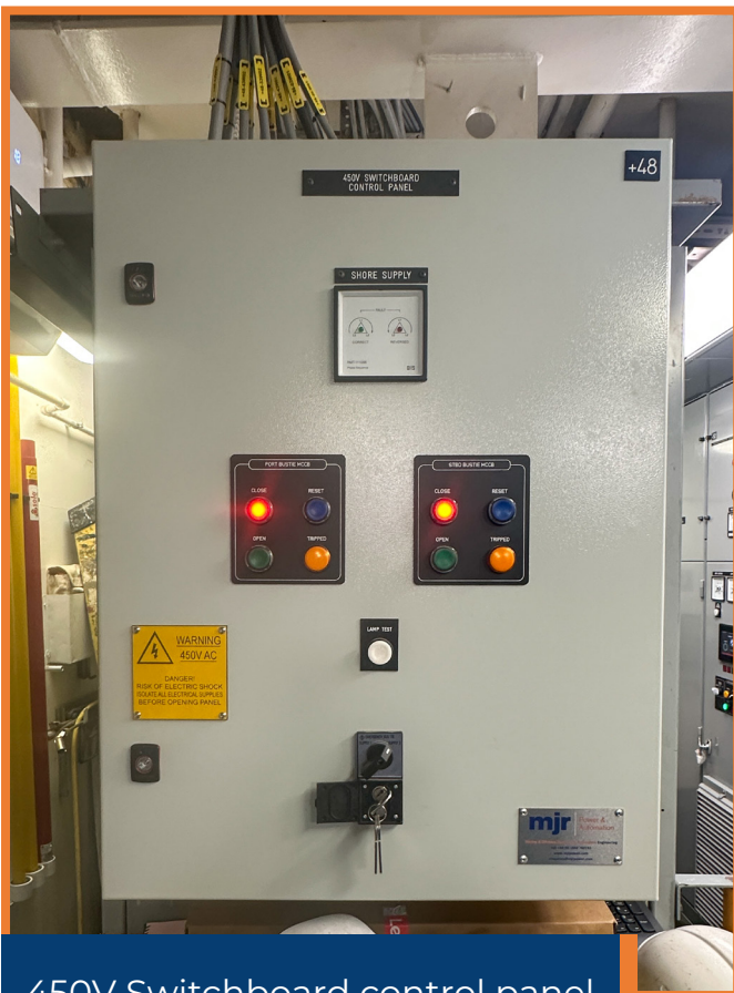
450V Switchboard control panel.
