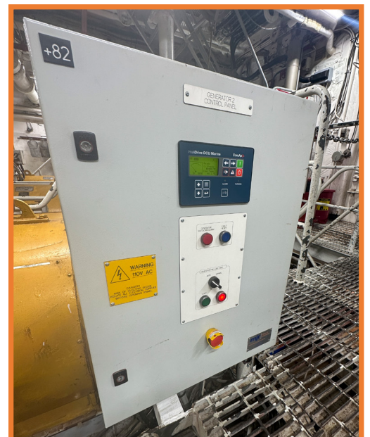
Four new generator control panels installed, one for each main generator.
