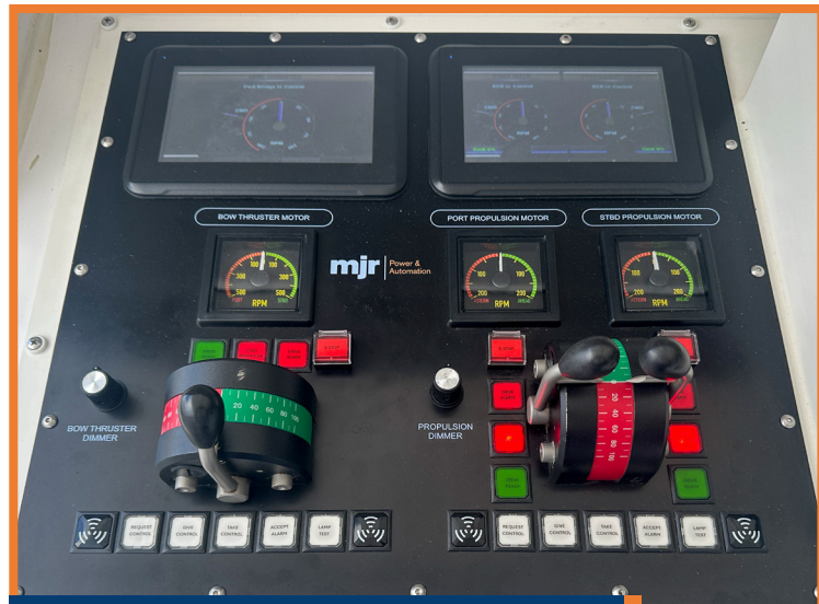
Bridge wing HMI panels for port, starboard and bow thruster motors.
