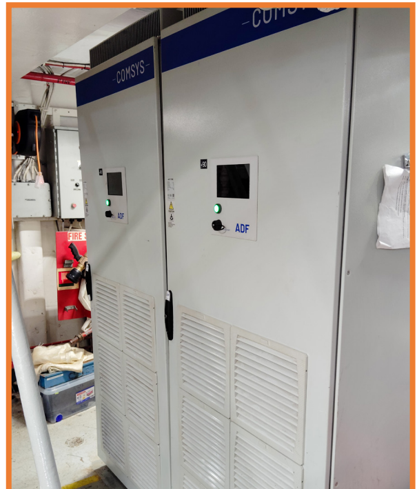
Two active harmonic filters for harmonic mitigation.
