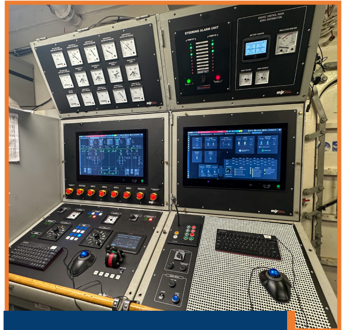
Engine Control Room Desk.
