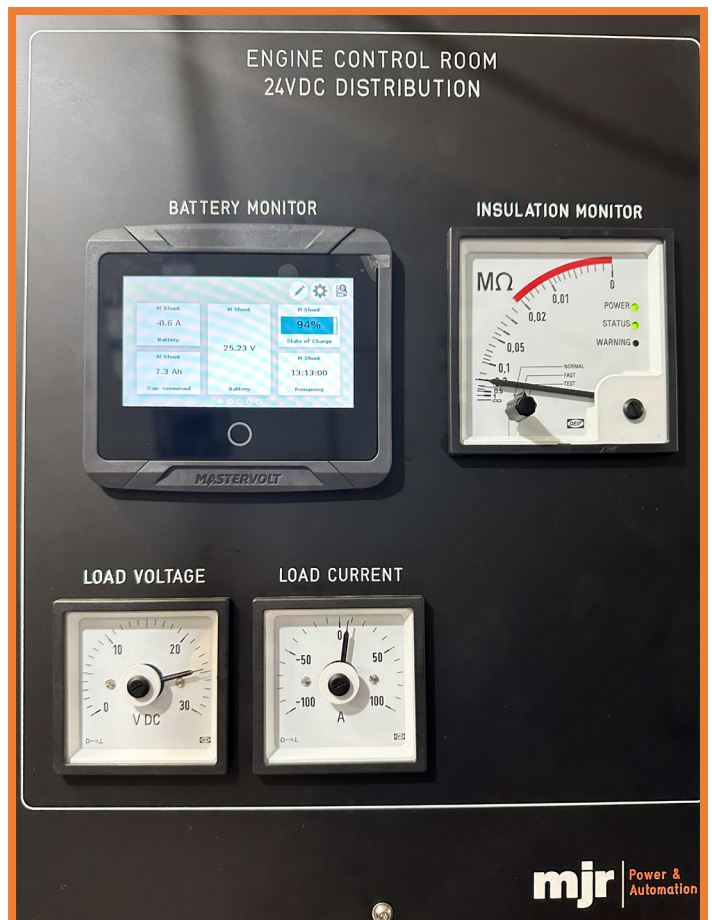
24VDC distribution display on the engine control room desk.
