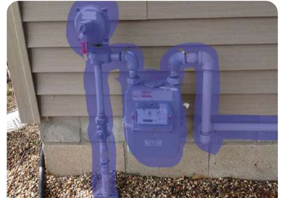
Zero-emission tag and proof of survey with no leaks found for a meter set scanned in about 8 seconds.
