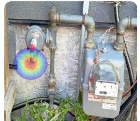
Residential meter set with a leak visualized by Laser OGI, scanned in about 5 seconds.
