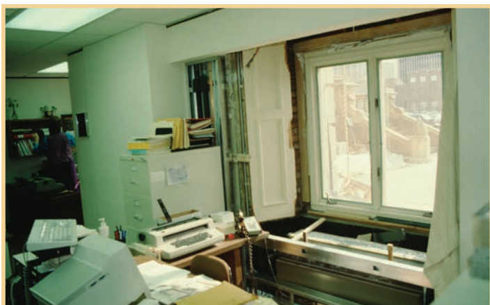
For many years Capitol offices contained a messy assortment of finishes and furniture that didn't date to any one historical period. Note the original woodwork around the modern window, which has been obscured at the top by a modern soffit.
