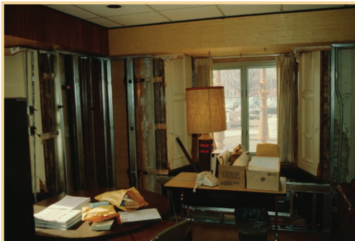
Prior to the restoration, the ground floor offices contained drywall built out from the walls, drop ceilings, fluorescent lights, and modern, inefficient windows.
