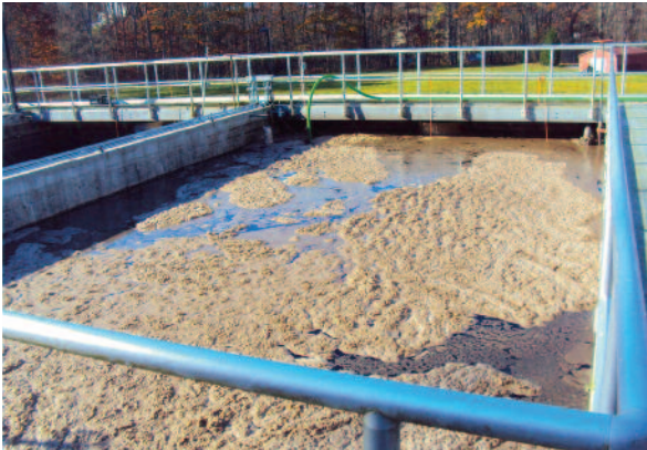
A green hose is used to transfer SBR decant to the digester tanks. No designed wastewater treatment process is currently conveying the supernatant between tanks.
