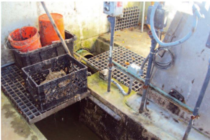
Automatic bar screen at plant headworks. Auto bar screen has not been operational and has only undergone minor repairs over the course of the last few years. Minor repairs do not maintain the unit in a consistent and operational state.
