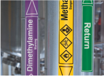
Pipe & valve marking
