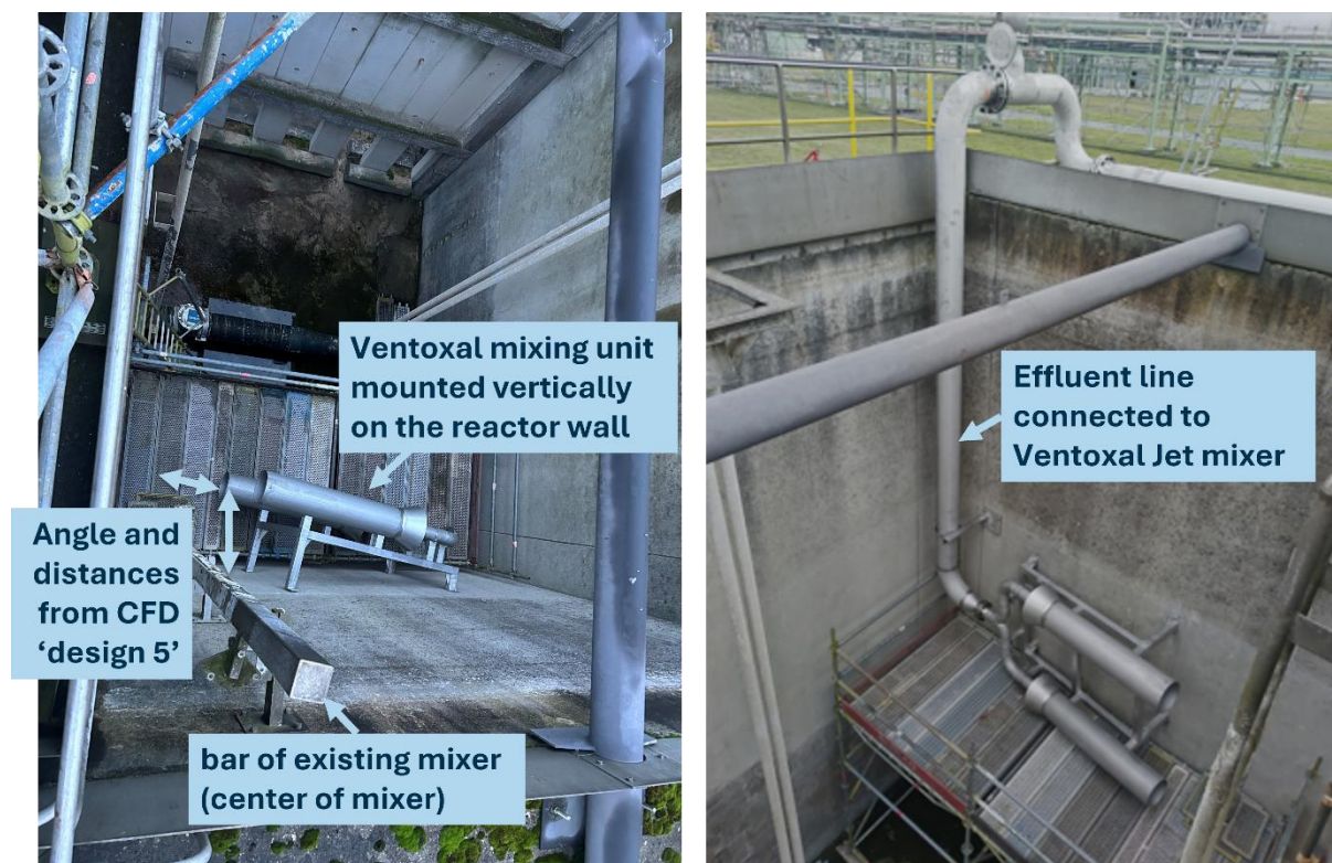
Figure 6: The Ventoxal mixing units were placed in accordance with the most optimal CFD scenario. This design, with a specific vertical placement of the mixing units, was expected to create minimal low-pH toxicity.
