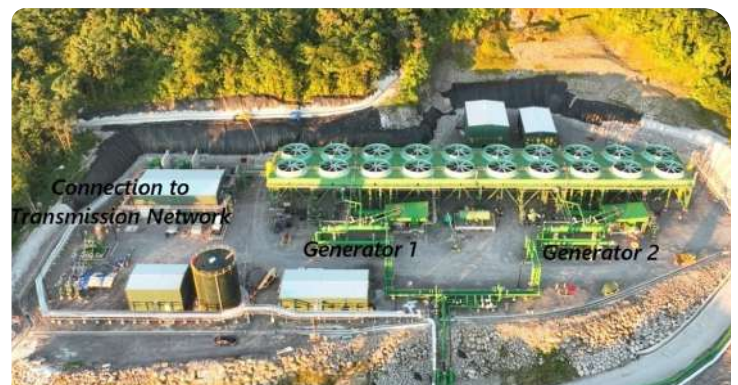
Figure 6: Dominica's Geothermal Plant (Source: Dominica Geothermal Development Company)
