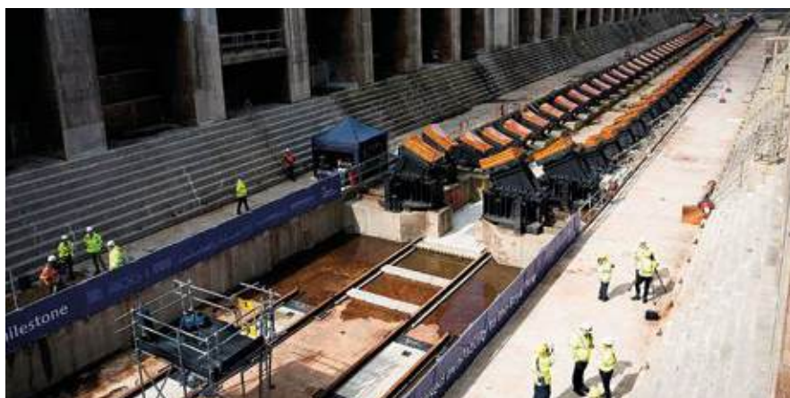
An empty No 9 Dock in HM Naval Base Devonport – home for HMS VICTORIOUS for the next few years whilst conducting her Deep Maintenance Period
