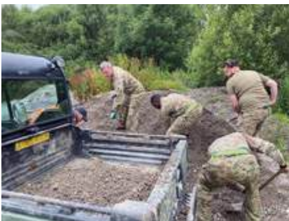
Cpl Peebles and the team moving 5 ton of gravel for the path repairs
