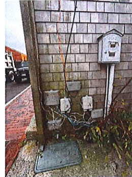
Fire Alarm Master Box
