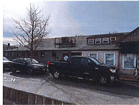
Roof Mounted Condensors
