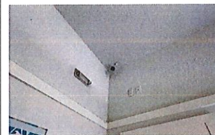
Existing Wireless Security System
