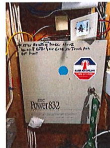
Existing Security System
