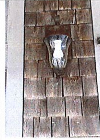
Exterior Light Fixtures
