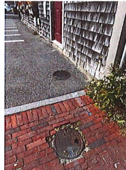
Domestic Water Service
