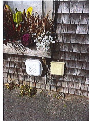
Telephone / Cable / Internet Service
