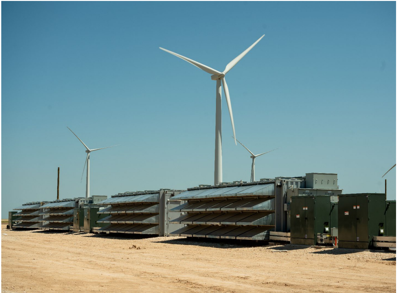
Photo of MARA's wind farm and on-site data center in Hansford County, Texas.
