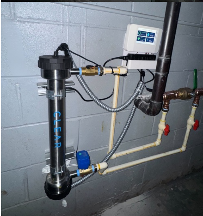
Example installations of Clear's UV LED system in this project.
