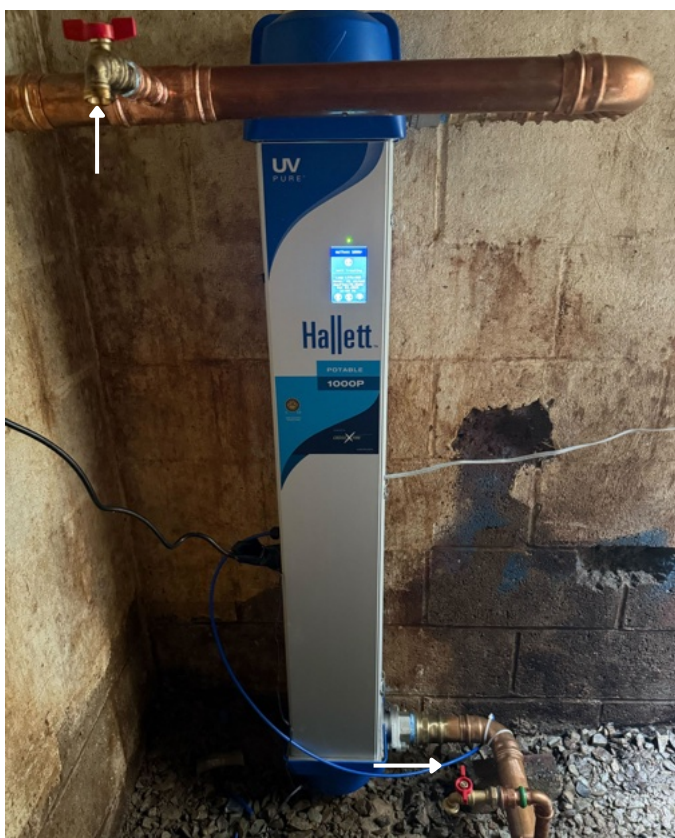
Figure 2. The UV system installed at the point-of-entry, with sampling ports (arrows) before and after the system.
