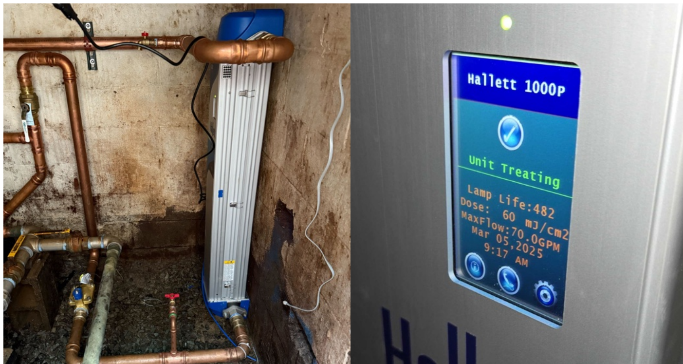
Figure 4. The installed UV system, showing the system display on the right.
