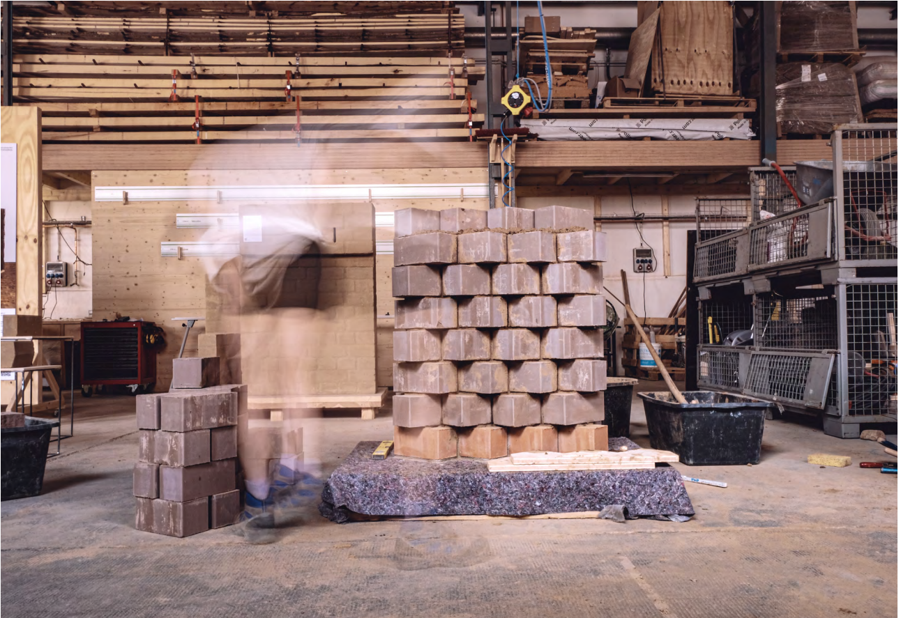
↑ Earth Block Masonry, Prototype © Bauhaus Earth, 2024 ← Production of Compressed Earth Blocks © Florian Janowitz, 2025
