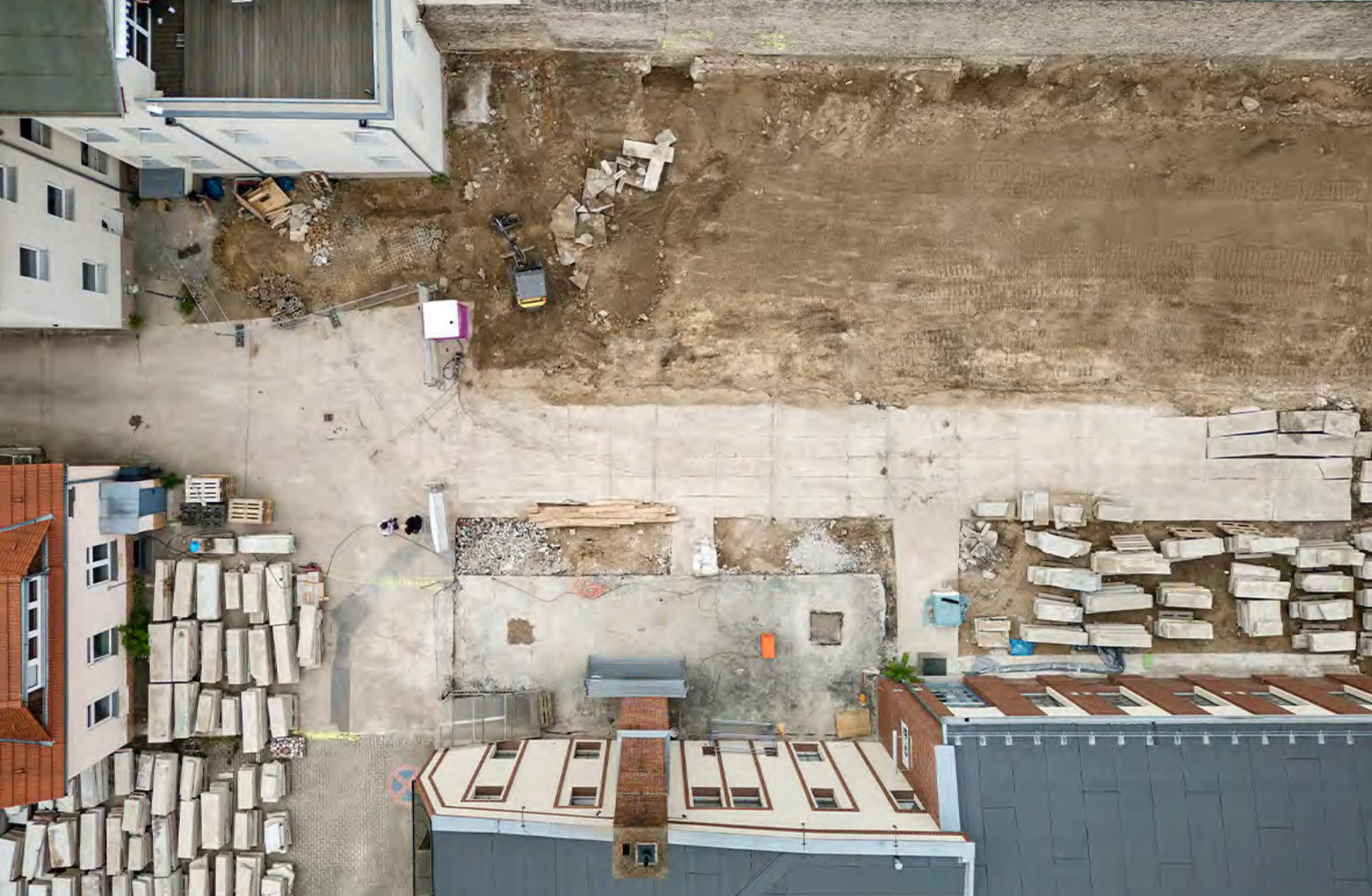
Re-use of the concrete foundation: aerial view of the B&O Bau construction site in Berlin-Weissensee, © B&O Bau; Photo: Jan Bitter, 2024
