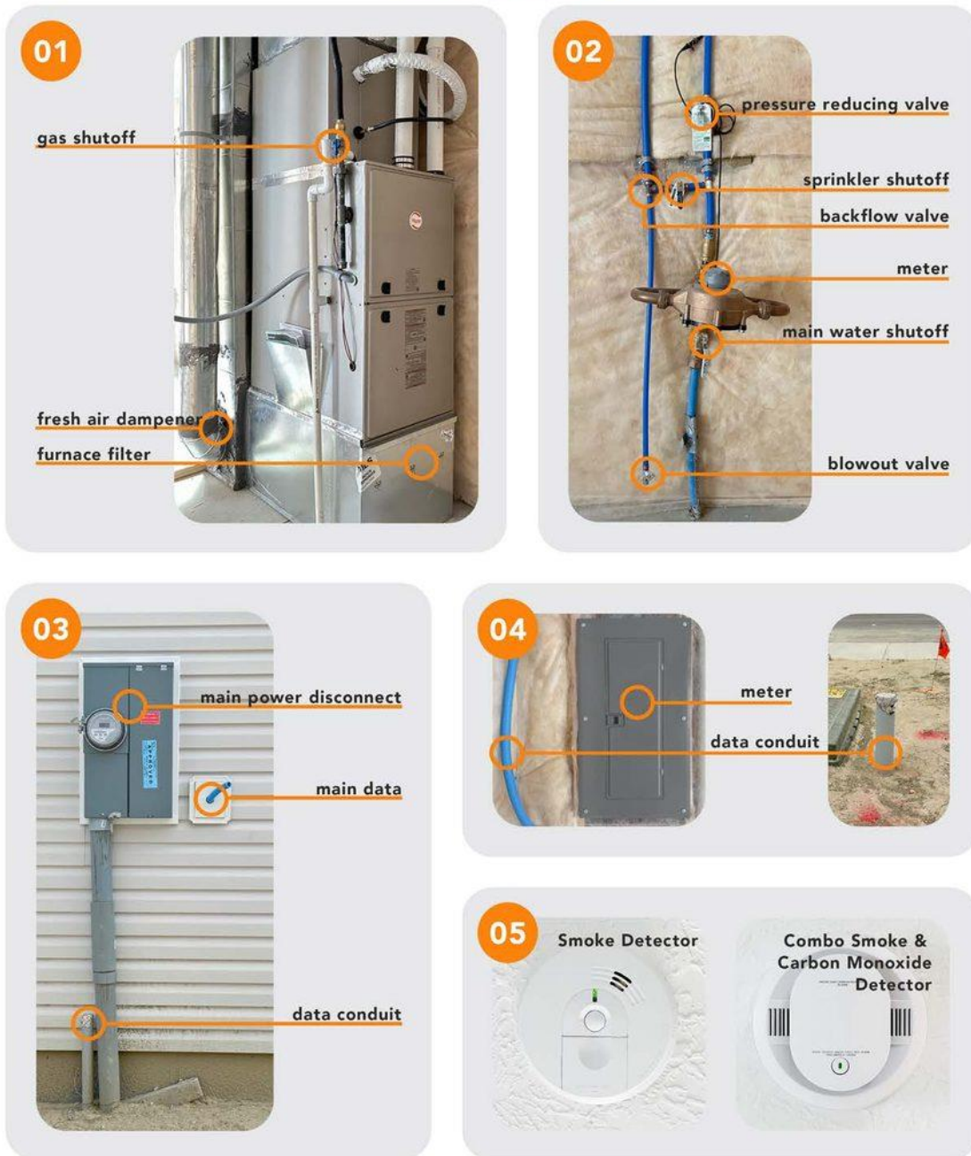
Reference Images 01–05: Gas shutoff, furnace filter, fresh air dampener, water valves, smoke detectors
