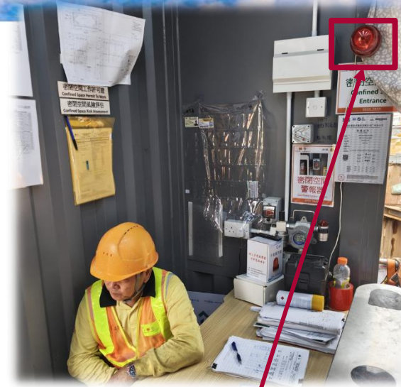
Audio-visual alarm light
