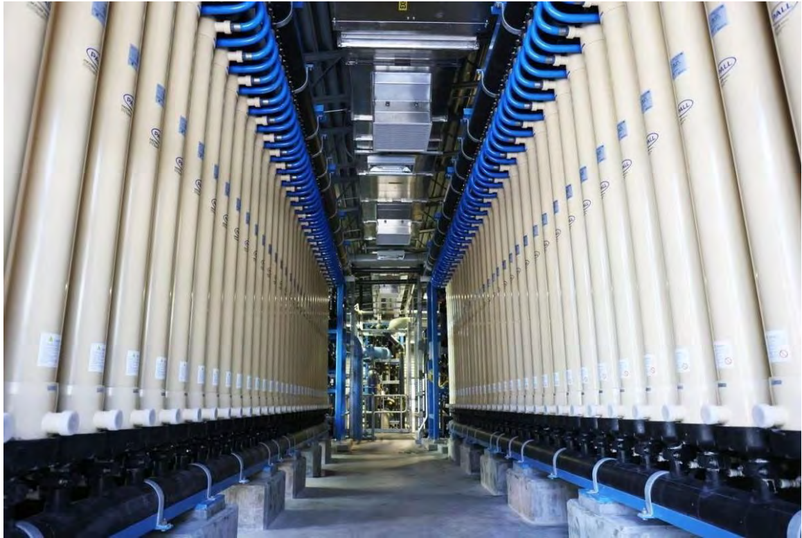
Outback Water Filtration Facility
