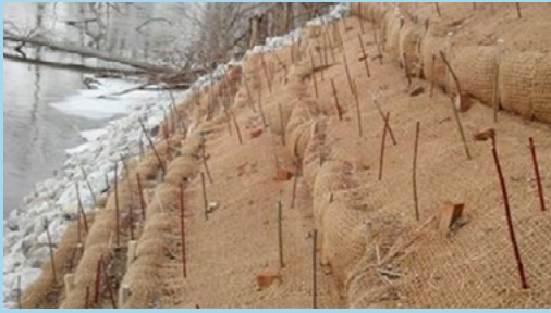
Slope stabilization using live stakes of dogwood & willow with coir blanket and slope interruption to control temporary erosion.
