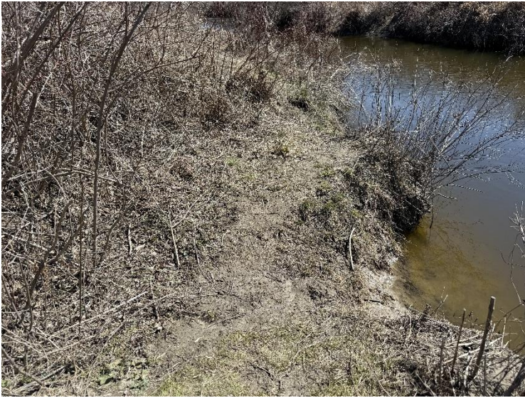
Photo 3. Bank erosion at existing launch location.
