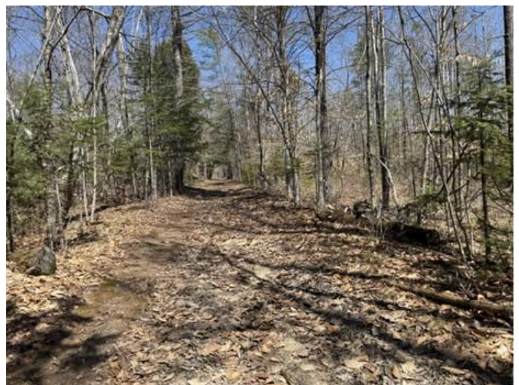
Photo 8. Trail conditions in Segments 6 and 7 are generally dry, with some existing gullies that require repair.
