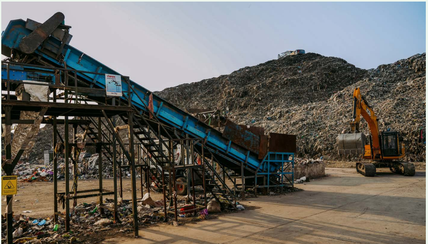
An infeed conveyor, where tipped material is conveyed for the initial sorting process.
