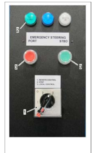
Motor Controller Cabinet
