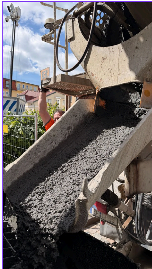
Caption: A biochar-concrete mix is being used in a slipform construction, marking the first time in the world this has been accomplished. Image used by permission of CarStorCon® Technologies.
