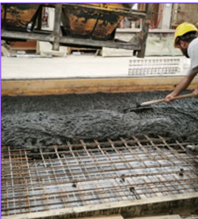
Caption: Concrete-biochar mix is being poured over a rebar form to create a precast wall element. Image used by permission of ecoLocked.
