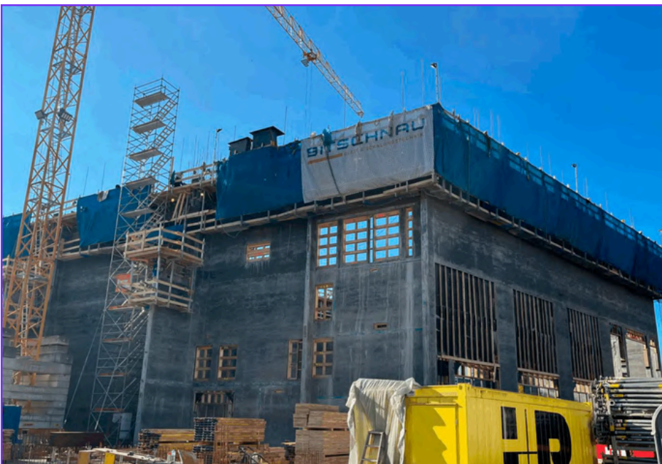
Caption: A biochar-concrete mix is being used in a slipform construction, marking the first time in the world this has been accomplished. Image used by permission of CarStorCon® Technologies.
