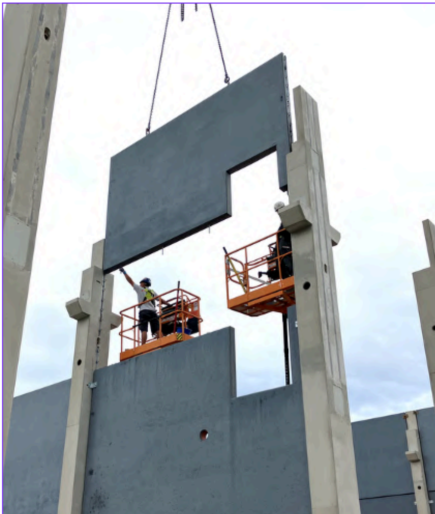
Caption: Precast concrete walls made with biochar admix from ecoLocked are being installed in Kemnath, Germany with construction and engineering company Markgraf. Image used by permission of ecoLocked GmbH.
