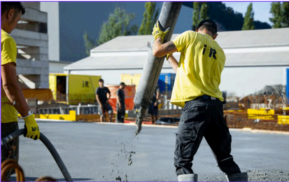
Caption: A biochar-concrete mix is being pumped to build the foundation of the new energy plant at Wallenmahd. Image used by permission of CarStorCon® Technologies.
