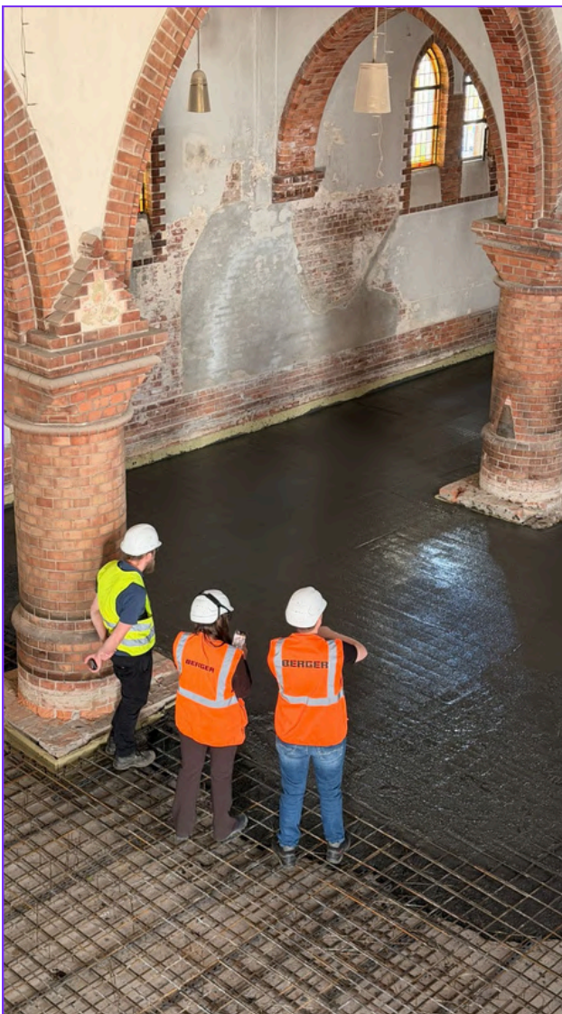
Caption: A biochar-concrete mix is being pumped to build the foundation of the new energy plant at Wallenmhd. Image used by permission of CarStorCon® Technologies.
