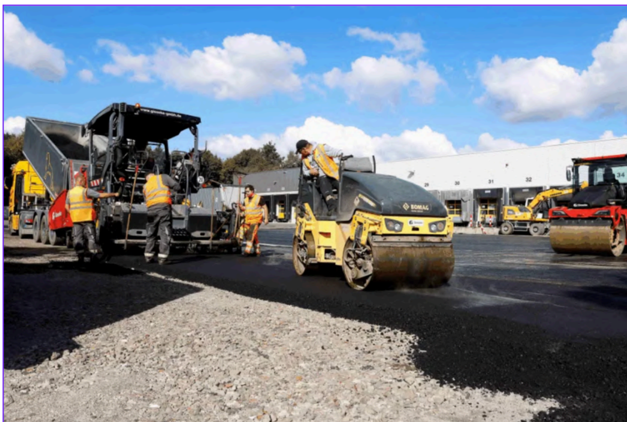
Caption: Carbon neutral asphalt is being laid by Gieseke GmbH. Image used by permission of Gieseke GmbH.
