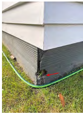
Damage to fibre cement.
