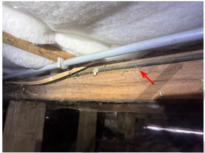
Example - old non compliant power supply wiring.
