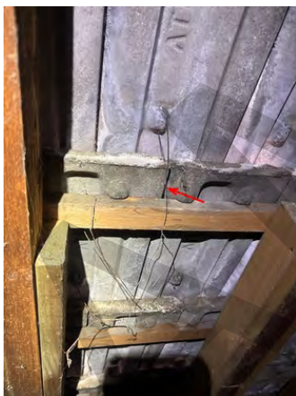
Example - many metal tile ties need re-attaching.
