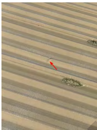
Minor dent to roof.
