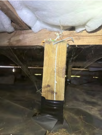
Pile is split through and z nail detached. This has been glued together.
