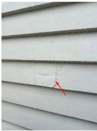
Rot under the penetration patch. Replace board here.
