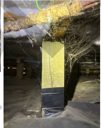
Monitor splitting on this pile.
