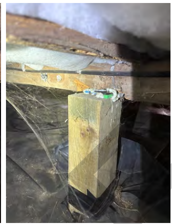
Pile not strapped in this side and not sitting properly under bearer.
