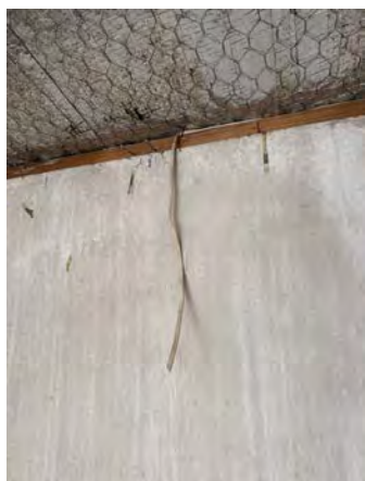
Disconnected power for lights.
