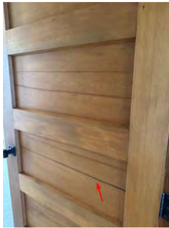
Example - many internal doors have some splitting to the panels from age.
