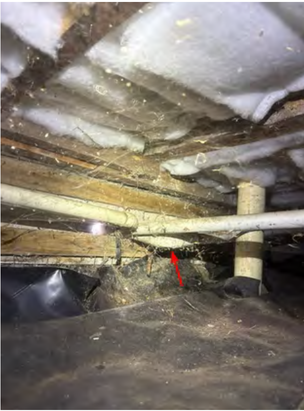
Bottom waste is running up hill. This needs adjusting.
