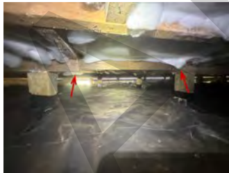
Bearer not properly supported on piles here.
