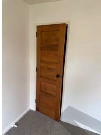
Striker plate needs a slight adjust.
