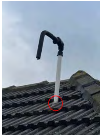
No flashing installed to hot water boiler over pipe penetration.
