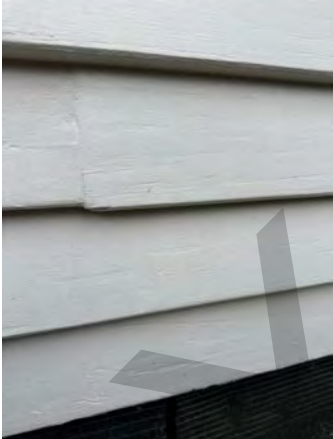
Close up example of typical weathering to boards throughout.
