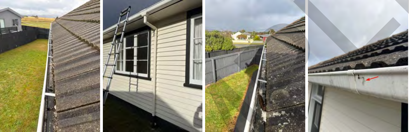
Crack in gutter.
