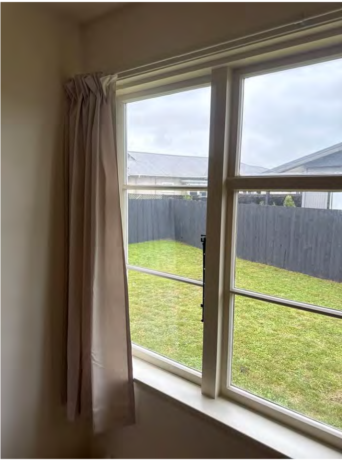
Window needs an ease.
