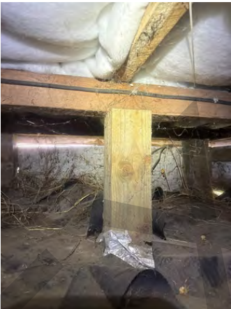
Pile needs strapping.
