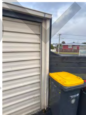
General denting to down pipe.
