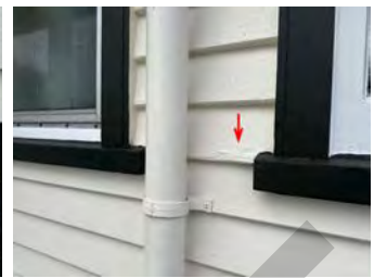
Minor rotting to board.
