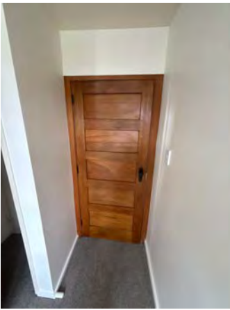
Some splitting to door panel. Striker plate has been notched out to a rough standard and the latch return on the handle is weak.
