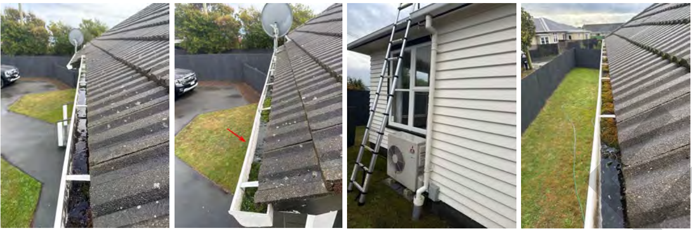
Some sagging to gutter above main entryway.
