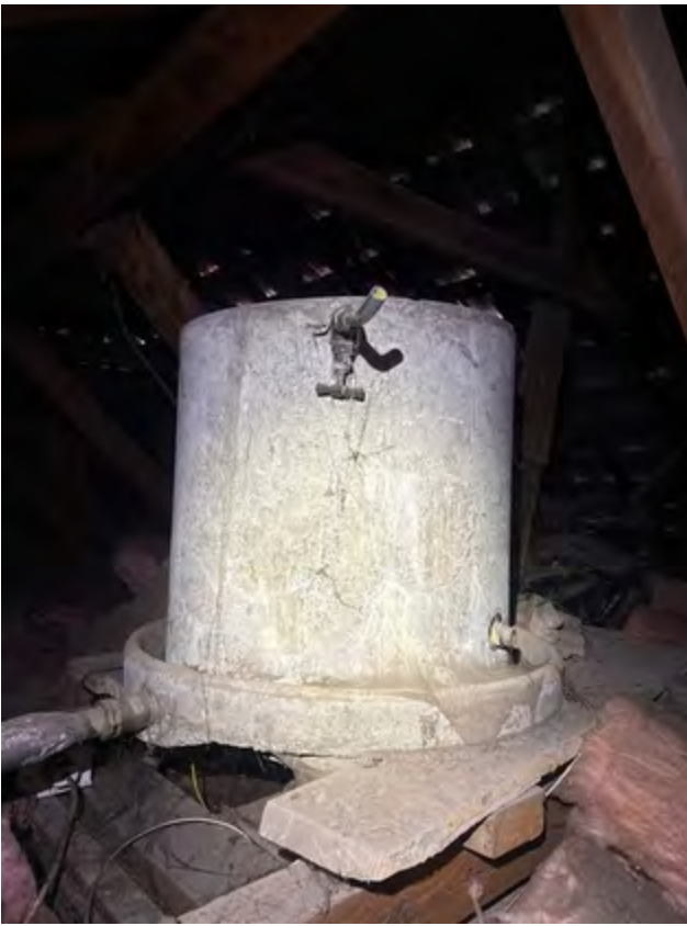
Obsolete header tank is best removed from the ceiling cavity.
