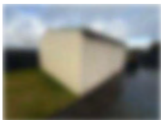
Some denting and typical light corrosion to garage doors and flashings.
