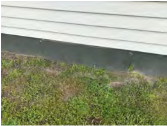
Some chips to sheet that is used as the sub floor access.
