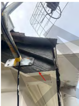
Example - some paint degrading in areas.
