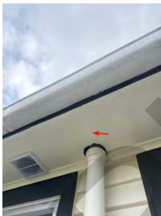
Crack in soffit.
