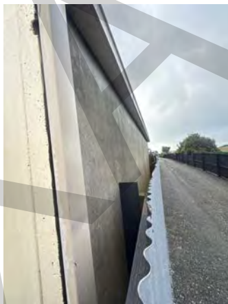
Rear wall could be painted.
