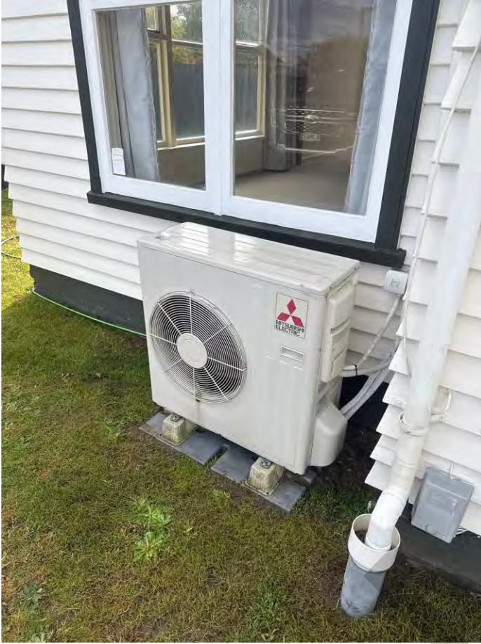
Some surface rust to condenser enclosure.
