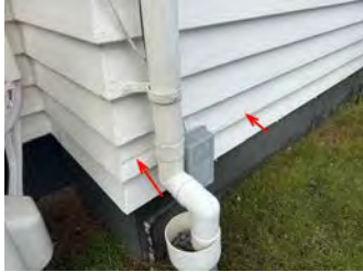
Split and possibly some rot to board.
