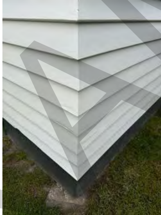
Several split and rotten boards to the northern corner.
