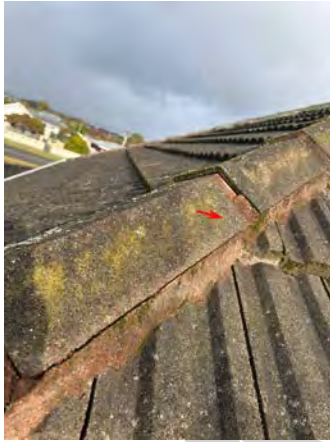
Minor crack to tile on eastern hip. This is best replaced.
