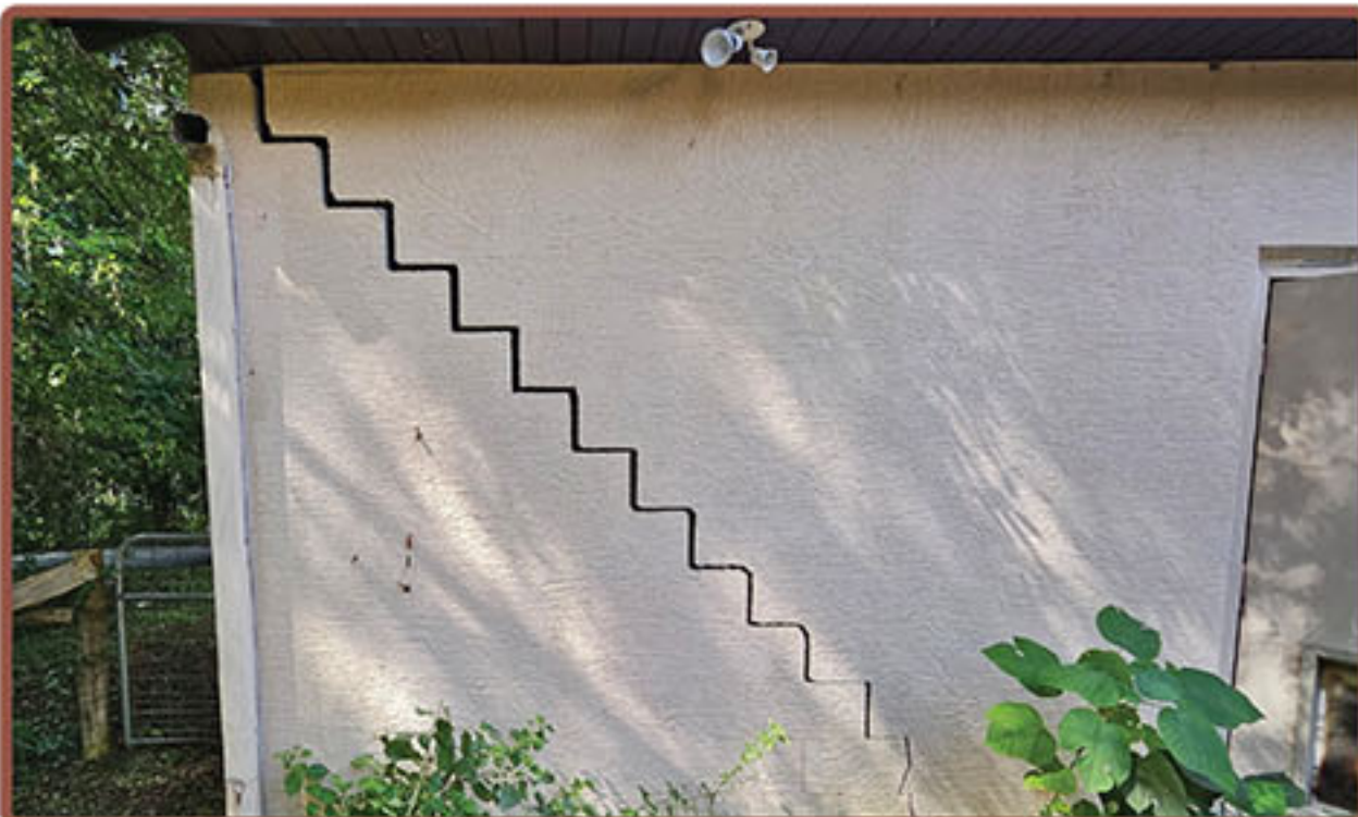
Diagonal, horizontal, and vertical cracks can be signs of settlement.
