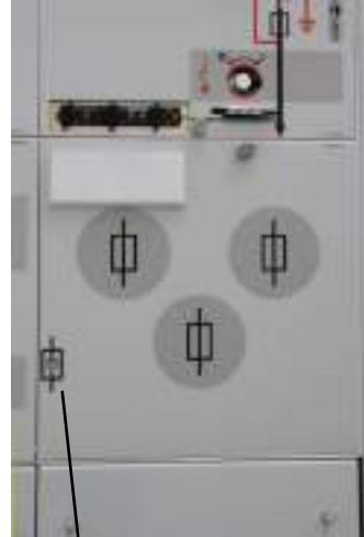
1. Indikator for utløst sikring.
