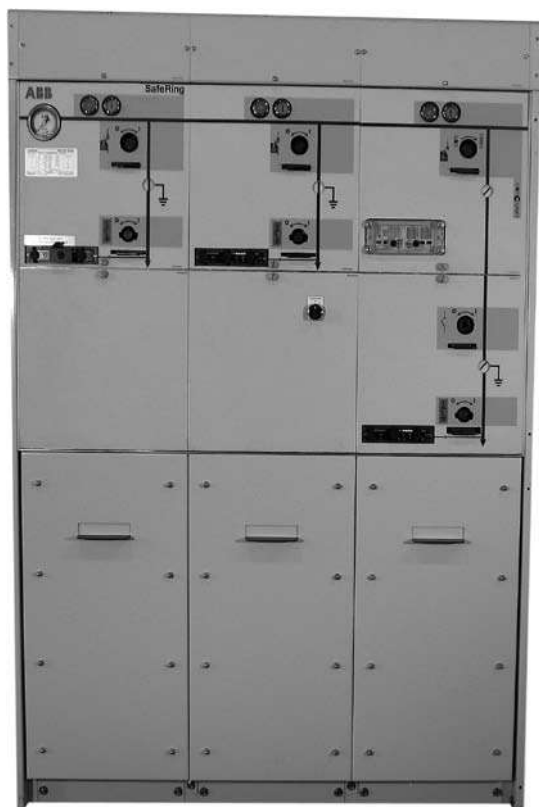
Top entry box low voltage cables
