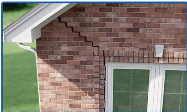
Stair step, horizontal, and vertical cracks can be signs of settlement.
