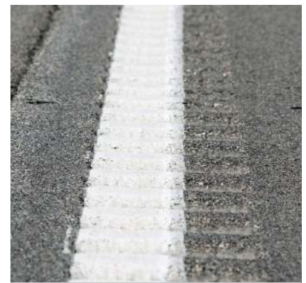
Example of an edge line rumble stripe.
